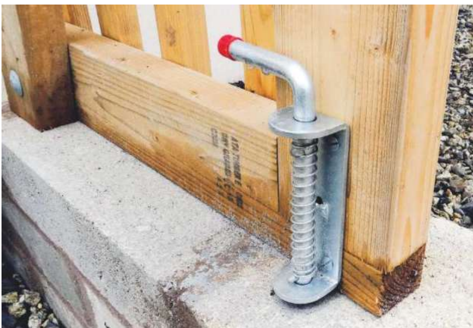
I used two standard fixings here: the bolts stop the logs pushing the sides out...
